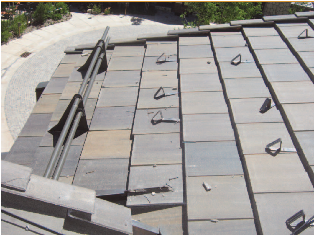
Photo 9 – Snow damage of the cleats and tiles due to build-up of ice and snow behind the retention bars. The clips do not have structural capacity to resist the loads imparted from the sliding ice and snow.
