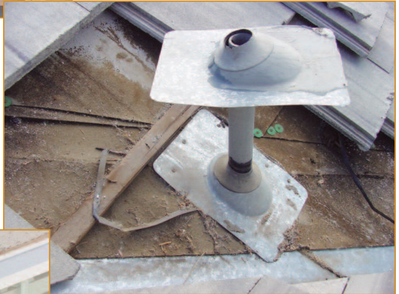
Photo 4 – The integration of penetrations through the roofing requires that the roofing subcontractor work with the plumbing subcontractor to ensure that the lower flashings are integrated in a shingle-lapped manner and sealed, and that the upper flashings are integrated with the tile and sealed. In this case, the penetration near the valley is a problematic detail that should not occur. Simply put, keep holes out of valley construction.
