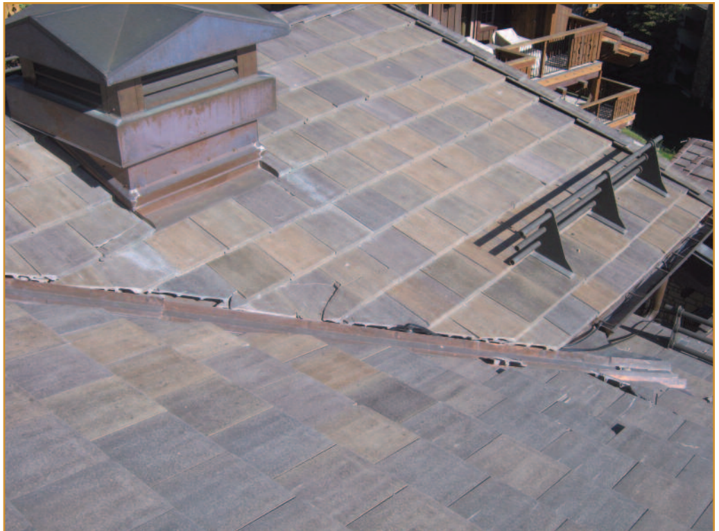
Photo 1 – Damage due to snow and ice accumulation in the valley area. The edge of the tile and the supporting valley flashing must provide structurally sound products in this area.
