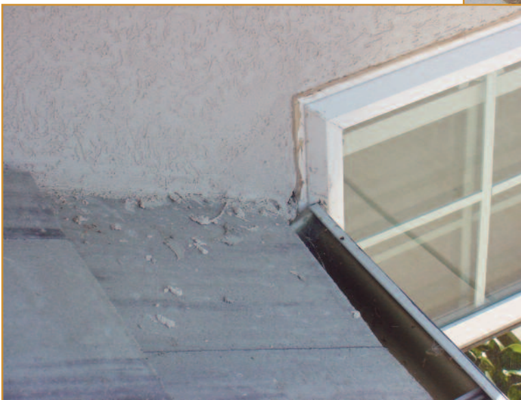
Photo 5 – The integration of the flashing from the roofing and the sidewall cladding is extremely important. The roofing subcontractor must ensure that the roofing felts, waterproofing, continuous flashing, and diverter flashing are all coordinated so they lap properly. A situation like the one in the photograph above should be brought to the attention of the designer of record. The window is damaged due to the location of the gutter, and because without flashings, water is directed into the jamb of the window. Contractors and subcontractors should not proceed with their work until such situations are fully resolved.
