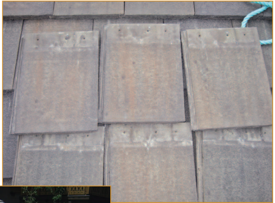
Photo 10 – The installer must determine the proper fastening and location. This as-built condition shows the nail size chosen and that there are missing nails in the tile roofing.
