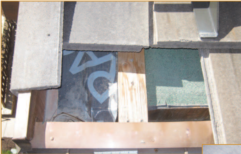
Photo 3 – The vertical batten prevents water in the channel from draining into the gutter below. The ice and water shield products must be properly integrated with the thermal envelope and the weather-resistive decking materials.
